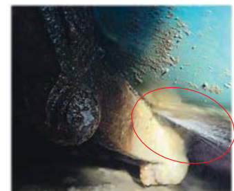
Leak at Pipe Joint
