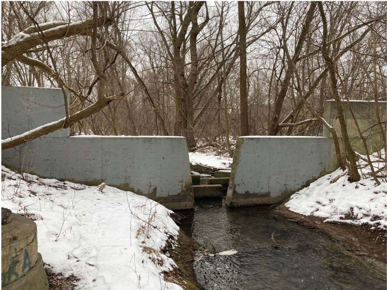
Figure 3-5 Typical On-Line Flow Control Weir (SWMF 24-2)
